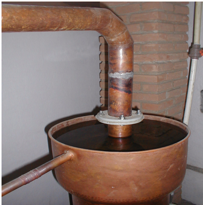
Fig. 12. Details of a cooling system on top of a hood-like column (CRD B, Paraty-RJ).
